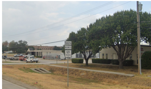
Drainage ditch and disconnected sidewalk segments.
