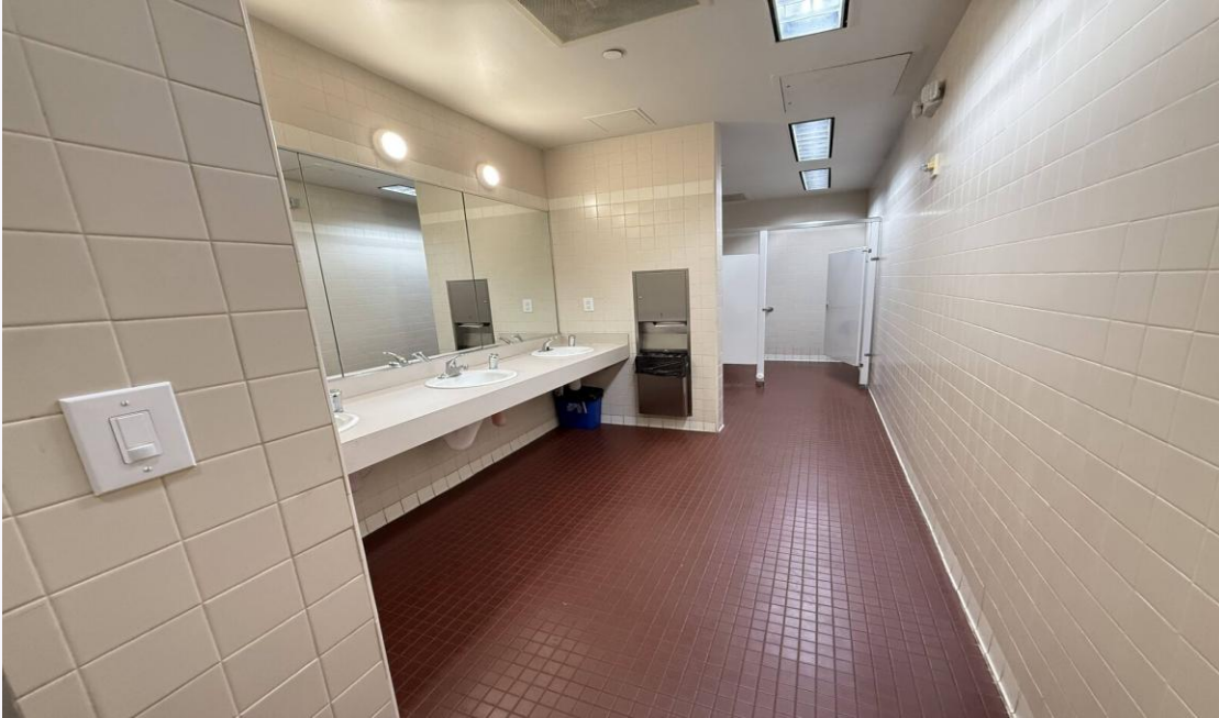
Current restrooms - original tile, fluorescent lighting, ADA compliance gaps.
