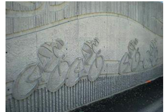
Formliners, as shown above, are an example of how community character can be integrated into infrastructure.
