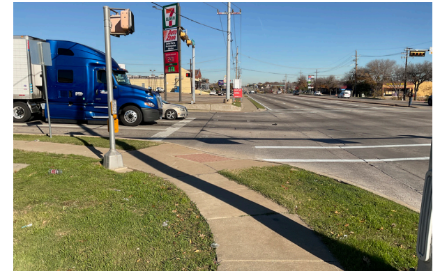
The intersection at Corporate Drive features faded crossing features and misaligned curb ramps, creating safety issues for pedestrians.
