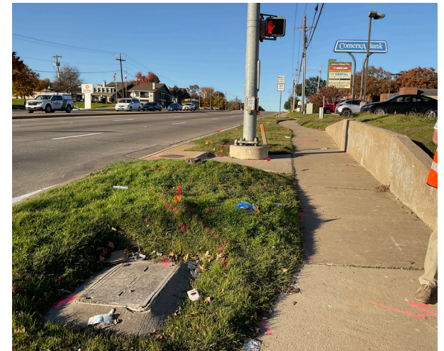
One of the pedestrian push buttons located at the intersection of Southwest Parkway is too far from the curb ramp.
