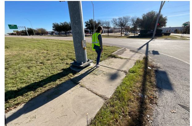
A lack of formal or deteriorating curbs causes safety concerns for drivers and pedestrians.
