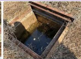
Open vault hazard 77
