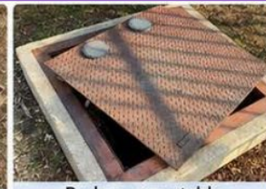
Broken or unstable access covers
