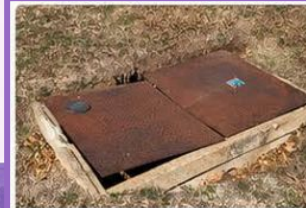
Damaged / misaligned lids
