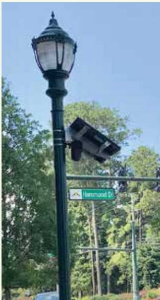
Solar & Existing Pole
