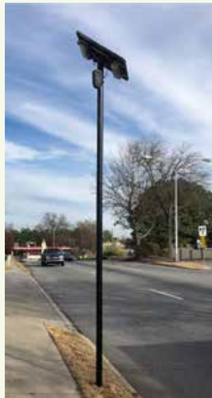
Solar & Flock Pole
