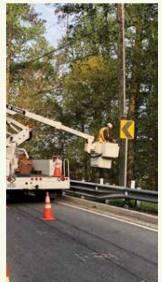
Electric & Existing Pole
